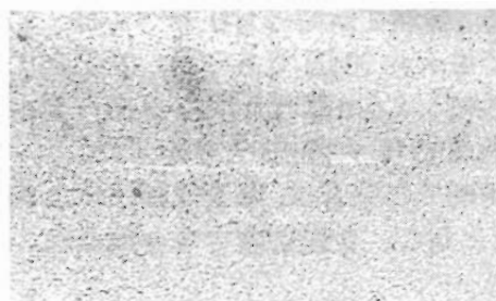
Photo 13 Metal Cutting Dust on Side Wall
