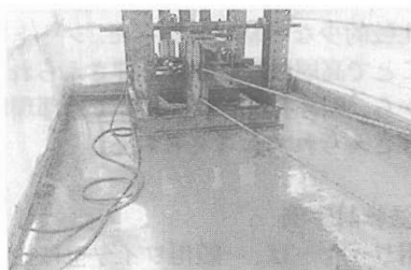
Photo 14 Slime of Mortar on the Floor
